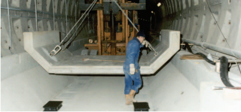
Floating-slab track, believed to be the most effective of all vibration countermeasures in new-build tunnels (Source: GERB, Germany)
